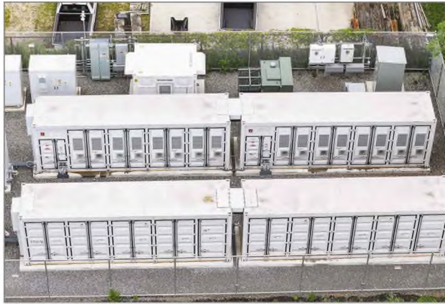
Battery storage units in Patchogue. There are 11 lithium-ion battery storage plants proposed for Suffolk.
